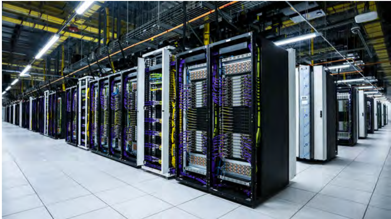
COLOSSUS II Facility in Memphis, Tennessee
